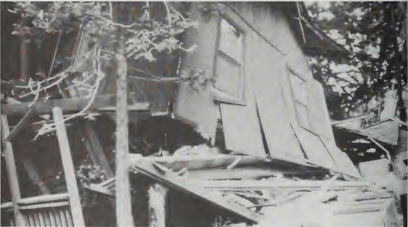
Collapsed residence in the Santa Cruz Mountains which is situated on the head of a landslide caused by the 1989 Loma Prieta earthquake. Geological investigations prior to construction may have revealed evidence of previous landslides, and informed the owner of potential risks at the site. Photo from Earthquake Engineering Research Institute.
